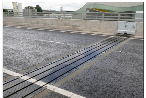
New installed TF expansion joint
