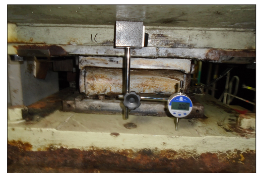
Bearing height monitoring of vertical deflection
